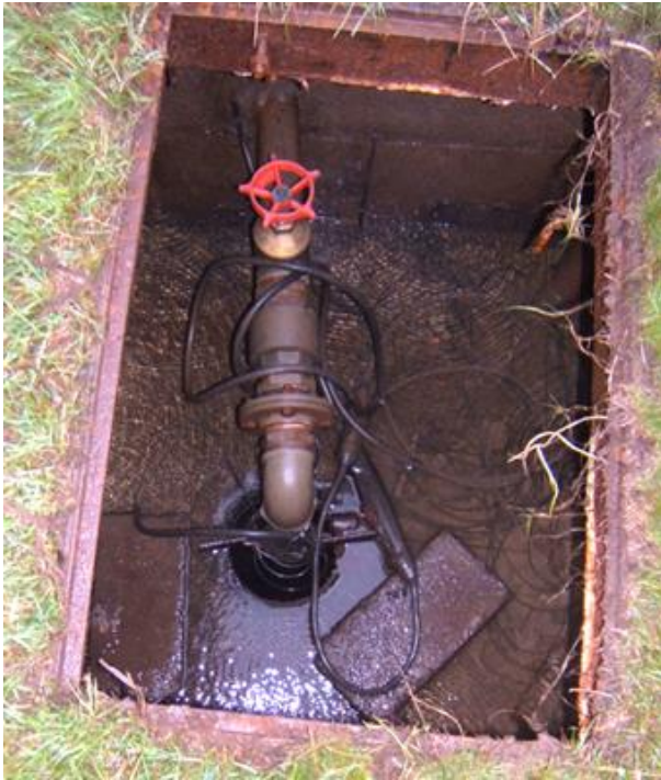
Figure 3 Poorly constructed wellhead with surface water entering top of the borehole (source: EPA).
