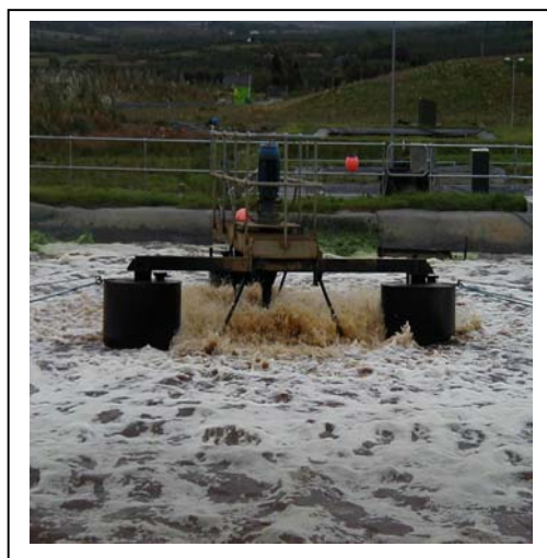
Gortadroma Landfill Aeration lagoon
